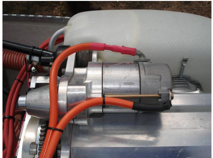
Cable Attached to End of Starter
